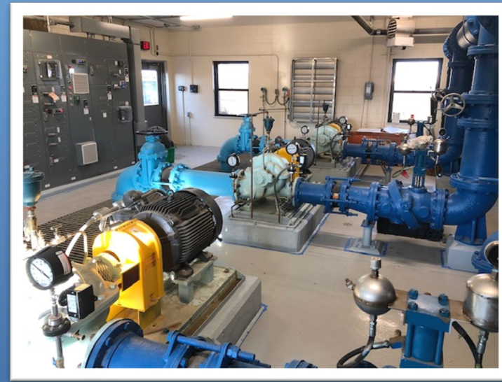
Newington Booster Station and Tank Aeration - 2019
