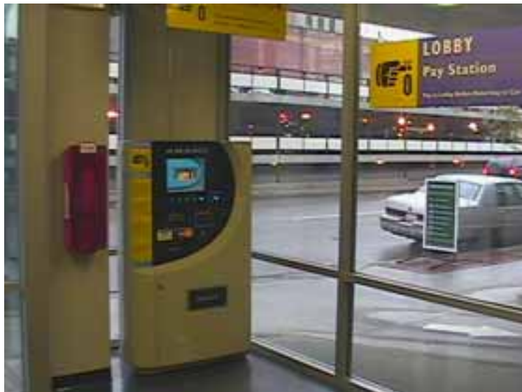
Typical Pay-On-Foot Station
