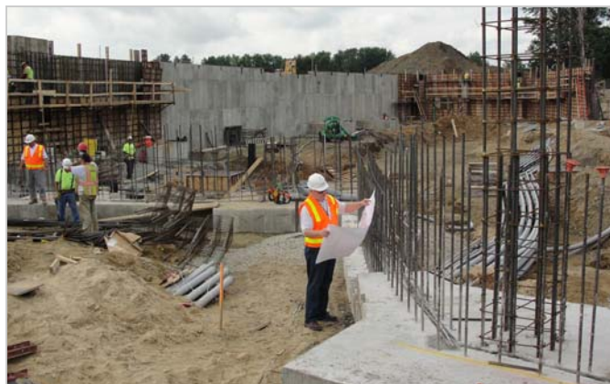
Chief Building Inspector Rick Hopley checks reinforcing at Service Federal Credit Union's new headquarters building
